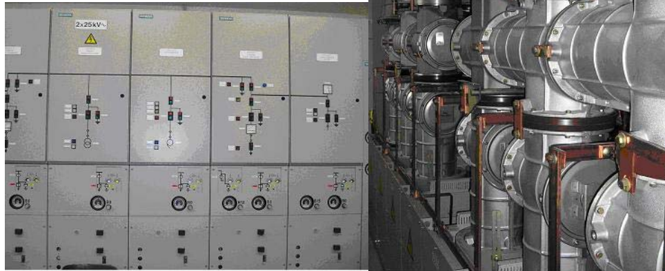
Picture 1 : 25 kV circuit breakers in interior type HV cells with a metallic casing & SF6 gas insulation
