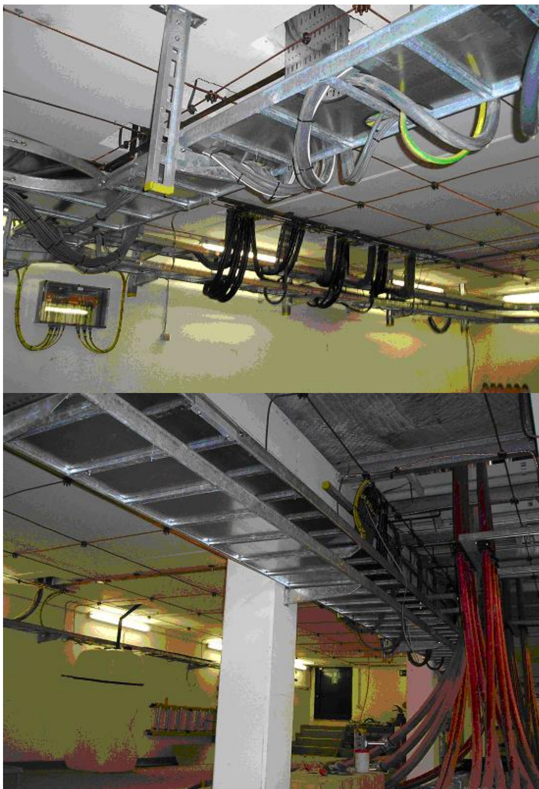
Picture 9 & Picture 10 : Installing metal plates at the bottom of cable ladders to transform them into cable trays
