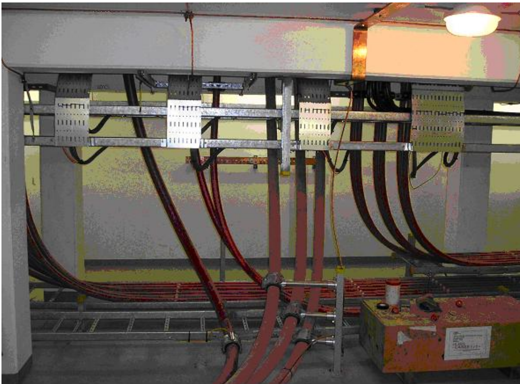
Picture 8 : Fitting a plate against cable trays to accompany the cables entering cabinets
