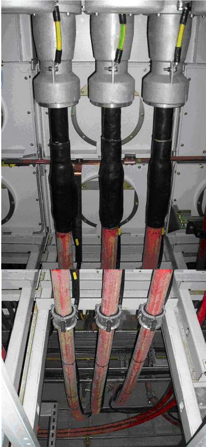
Picture 2: The shielding for the 25 kV cables is connected to the earth by insulated wires that are more than ten metres long.
