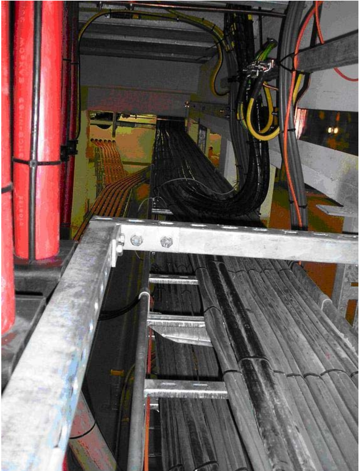
Picture 3 : The earthing wires are placed on cable ladders that also contain data and power cables.
