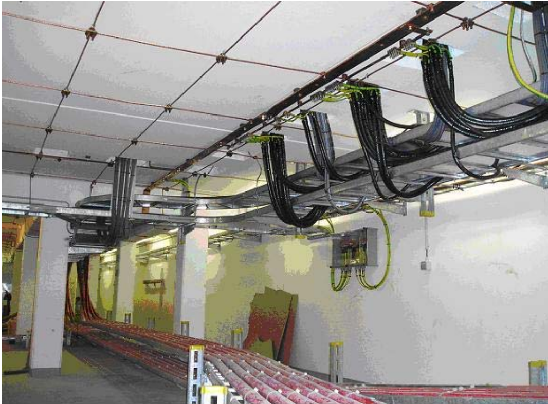
Picture 7 : Implementation of a meshed copper grounding grid suspended from the ceiling.
